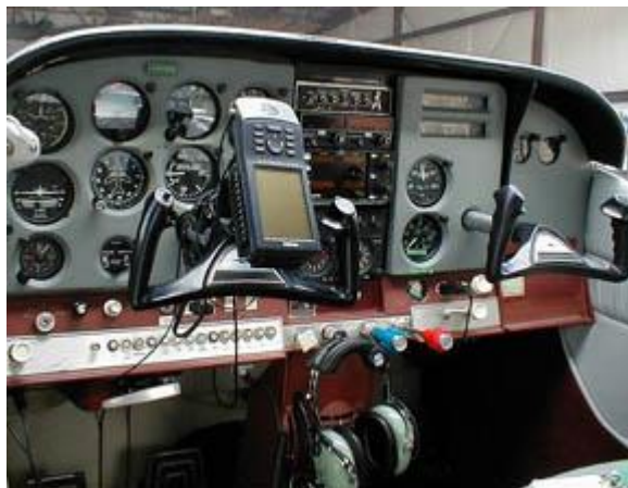
SA39-1823 glare shield installed in a 1965 Cessna 182 by Jack Fastabend of Richland, WA
