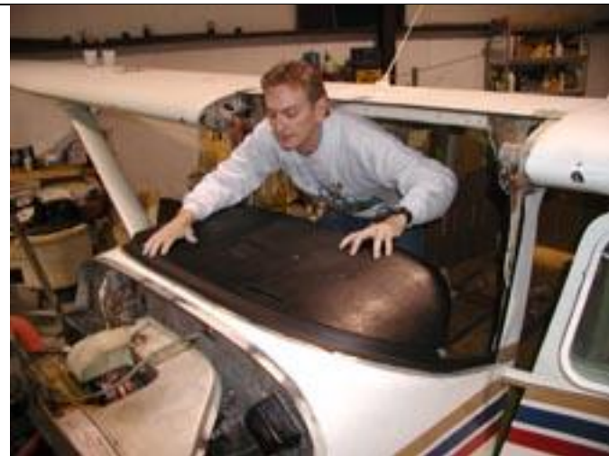
Step 3: Randy trial fits to see where glare shield needs to be trimmed. You can install the glare shield with or without the windshield installed.
