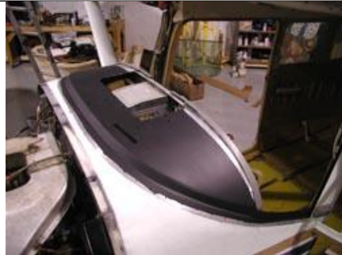
Step 1: The existing glare shield area was stripped and refinished with non-glare matte urethane.
